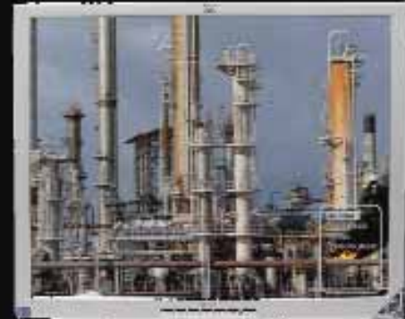
FlameVision 300 alarm simulated on a CCTV screen
