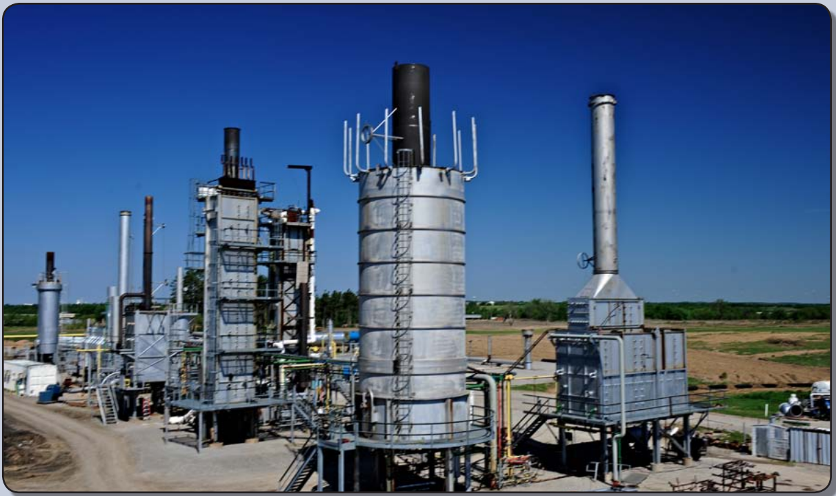
ZEECO Combustion Research and Test Facility
