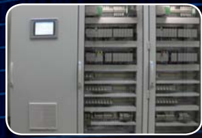
Burner Management System Enclosure
