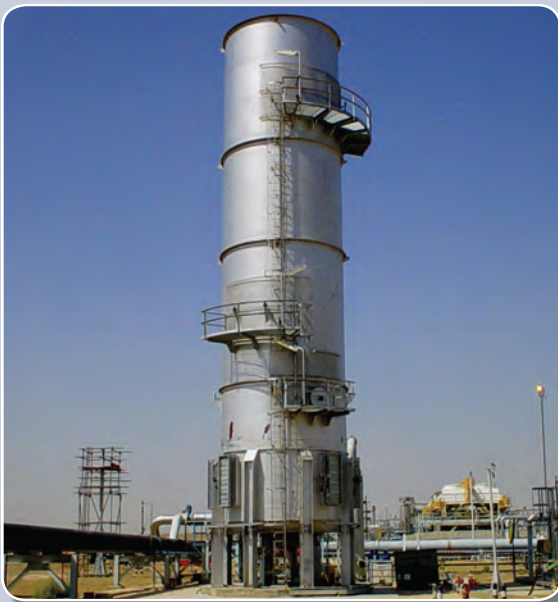
Natural draft SRU tail gas incinerator.
