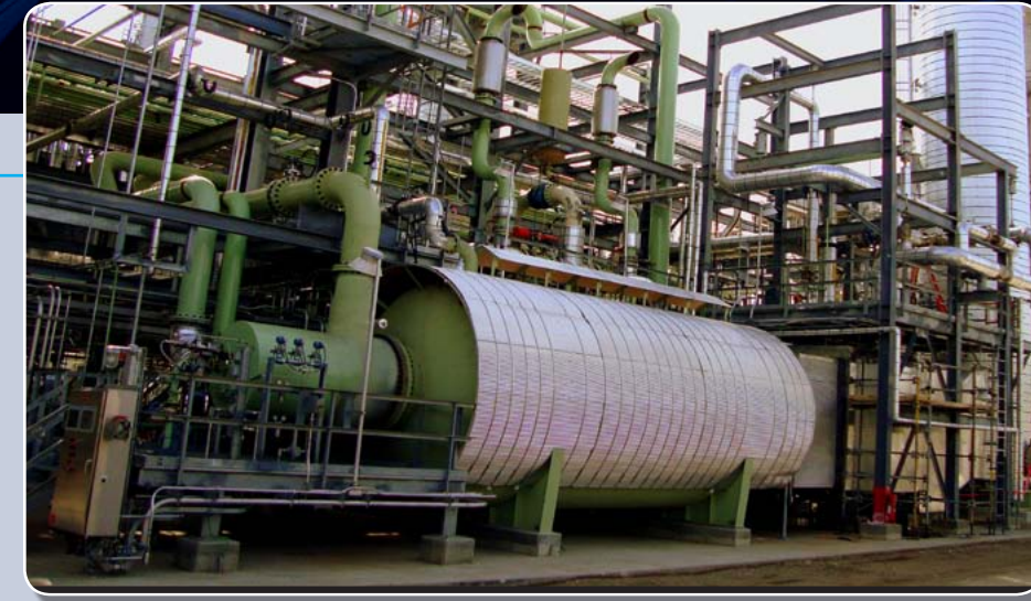
SRU Tail Gas Thermal Oxidizer with watertube style waste heat boiler
